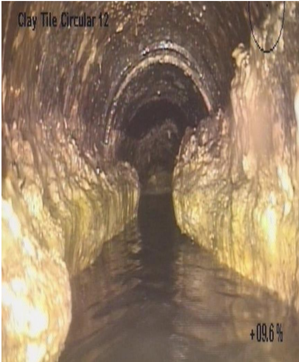
Recent picture from a camera in Onoway's sewerline on 48 th Avenue
